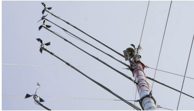
Figure 6. Photo of the sensors on the met mast
